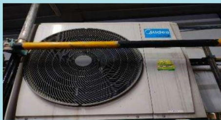
Inverter Air-con using at Site Office
