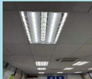
Photo showed the label for the TL5 fluorescent lighting using for site office
